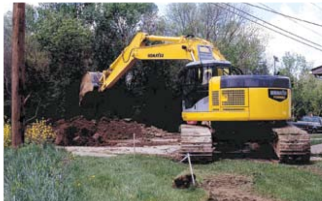
A leader in tight-tail-swing excavators, Komatsu offers nine compact models and construction-size units, including the PC308USLC-3, the industry's largest tight-tail-swing machine.
