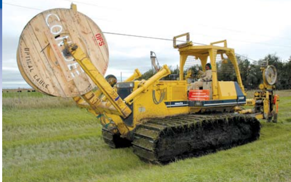
K&H Electric uses a specially equipped Komatsu D85PX-6 dozer to put optical cable in a trench near Conde, S.D.
