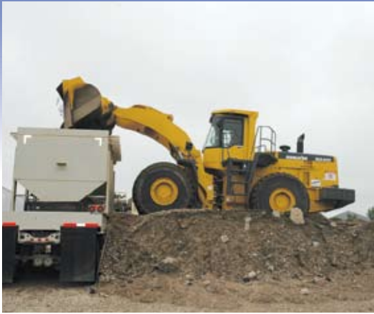
Using the company's new Komatsu WA500 wheel loader, a Turner Sand and Gravel operator carries materials at a recent job near Ehrhard.
