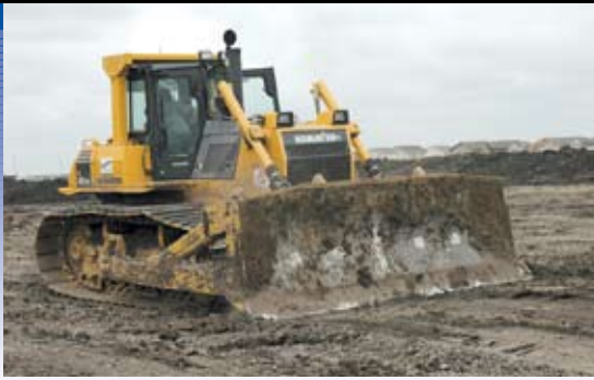
At the controls of a Komatsu D85 dozer, a Molstad Excavating Operator backdrags dirt in Grand Forks.
