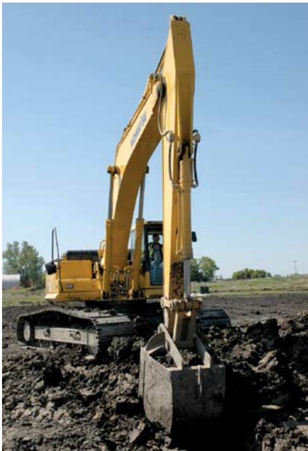
Foreman Allan Dunbar uses a Komatsu PC300LC-7 excavator to dig a trench on a jobsite in Mapleton.
