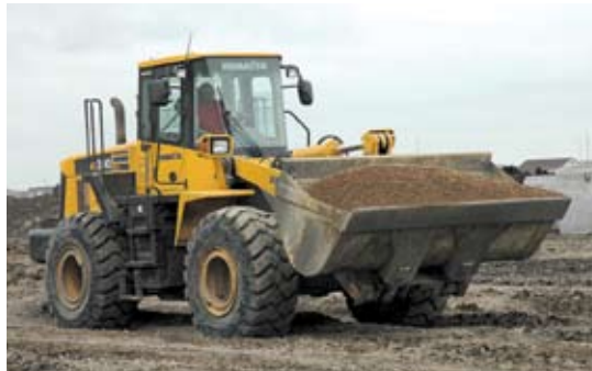
Using a Komatsu WA380-5 wheel loader, a Molstad Operator moves dirt at a housing development in Grand Forks.
