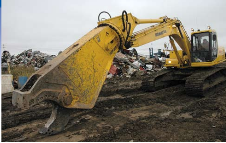
Hanson Auto Crushing & Trucking made its first Komatsu purchase, this PC250LC-6 excavator with a shear attachment, about four years ago.
