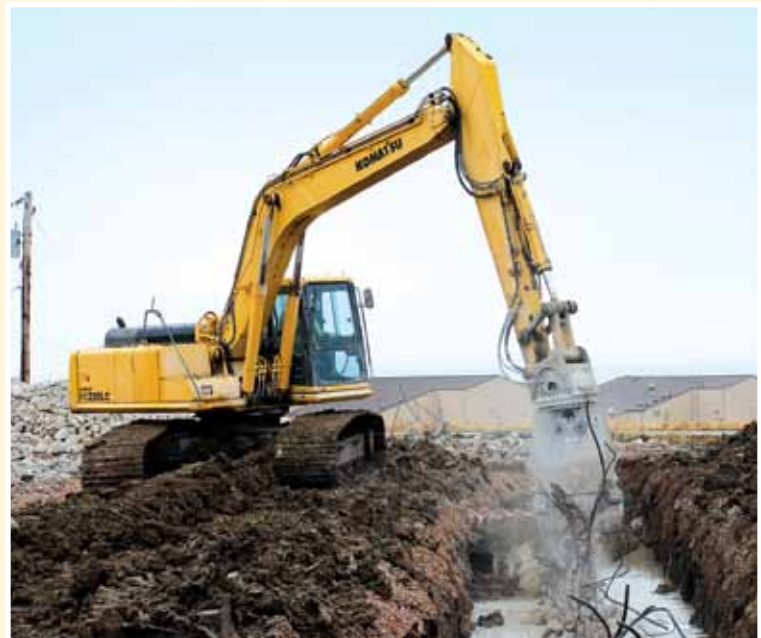
Many contractors use older Komatsu excavators for a variety of purposes, including such rugged applications as demolition.
