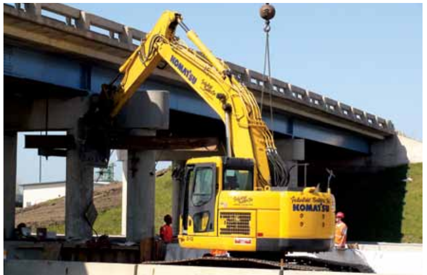
Industrial Builders relies heavily on Komatsu equipment, especially excavators, such as this compact PC228. “Our operators love the PC228s because they can work in a single lane of traffic without the worry of a big counterweight swinging into the other lane,” said Executive Vice President Donn Diederich.
