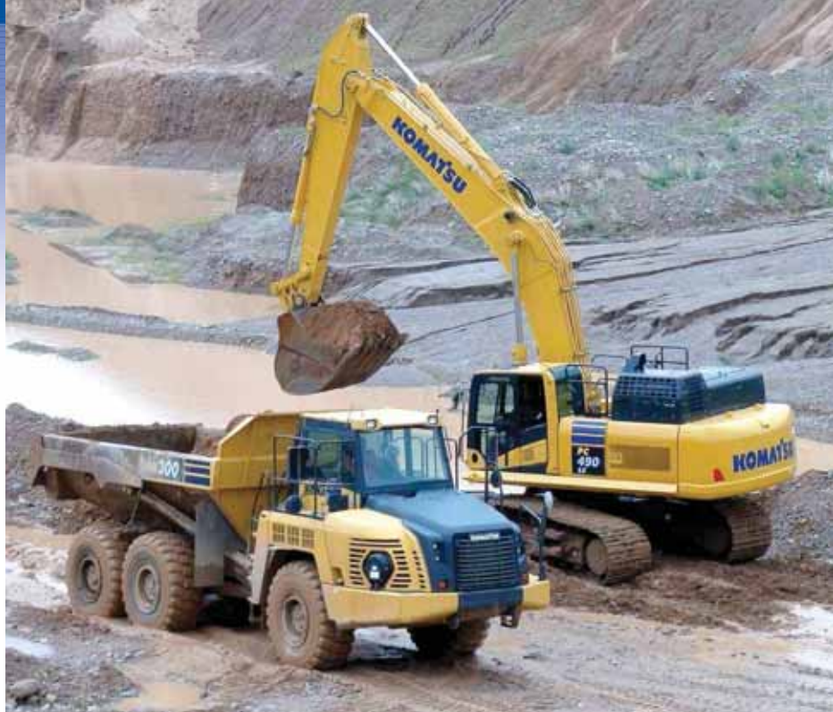
Komatsu's Chattanooga Manufacturing Operation (CMO) produces six sizes of hydraulic excavators, ranging from the PC210LC-11 to the PC490LC-11.
