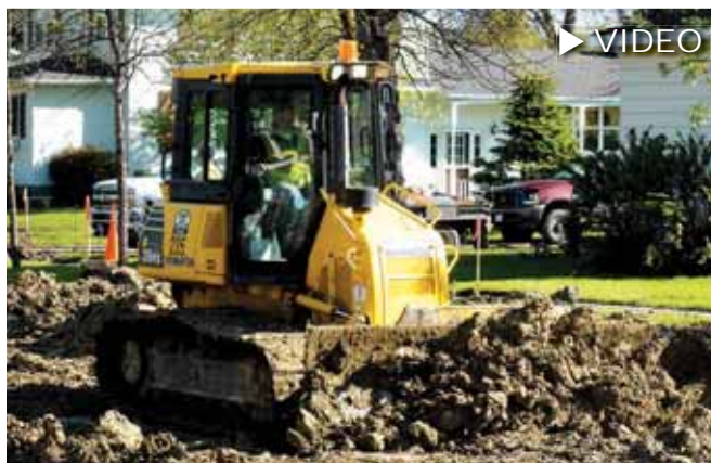
This Davidson Ready Mix & Construction operator backfills and grades with a Komatsu D39PX dozer on a jobsite in Warren, Minnesota.
