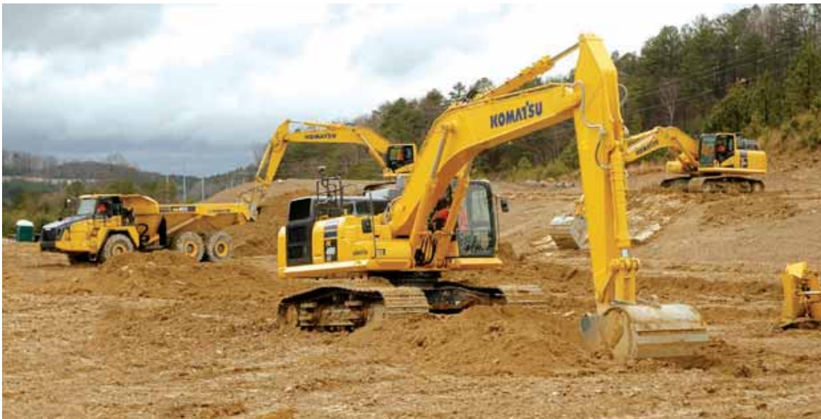
Komatsu's latest intelligent Machine Control excavator, the PC490LCi-11, was the main attraction at Demo Days. It is the world's largest GPS-integrated excavator on the market.
