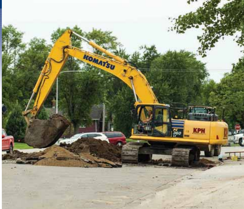
KPH is installing a water valve using a Komatsu PC360LC excavator at North Dakota State College of Science. “The PC360 is great for us because it is a very smooth, mid-sized machine,” said Vice President Patrick Hockett. “It gets the job done every time.”
