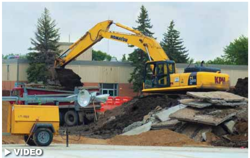
A KPH operator loads a truck with a ditching bucket after excavating sidewalks at North Dakota State College of Science.
