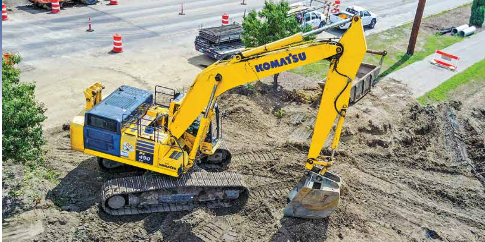
This crew from BEK Consulting uses a Komatsu PC490LC excavator to build a water basin at the intersection of University and 6th Avenue in Bismarck. "We love the Komatsu excavators for their fast cycle times and operator-friendly controls," said Vice President Lonnie Kern.
