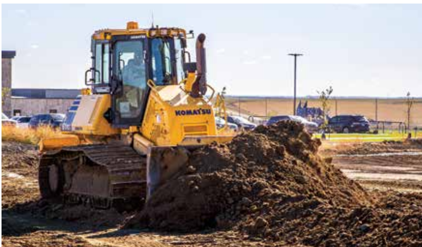
On a job site, an operator moves material with a Komatsu D61PXi intelligent Machine Control (iMC) dozer.
